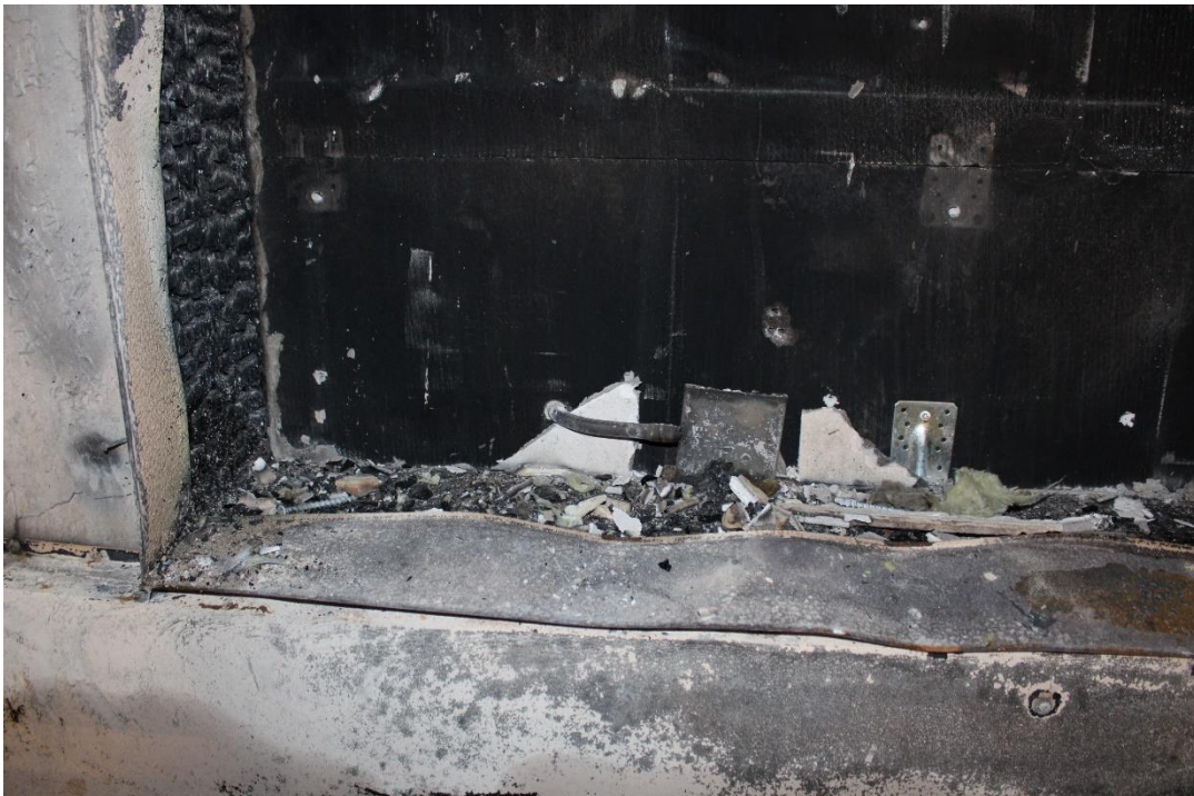
Photo No. 24 Test specimen after the test. Detailed photo of 1. Floor bottom.
