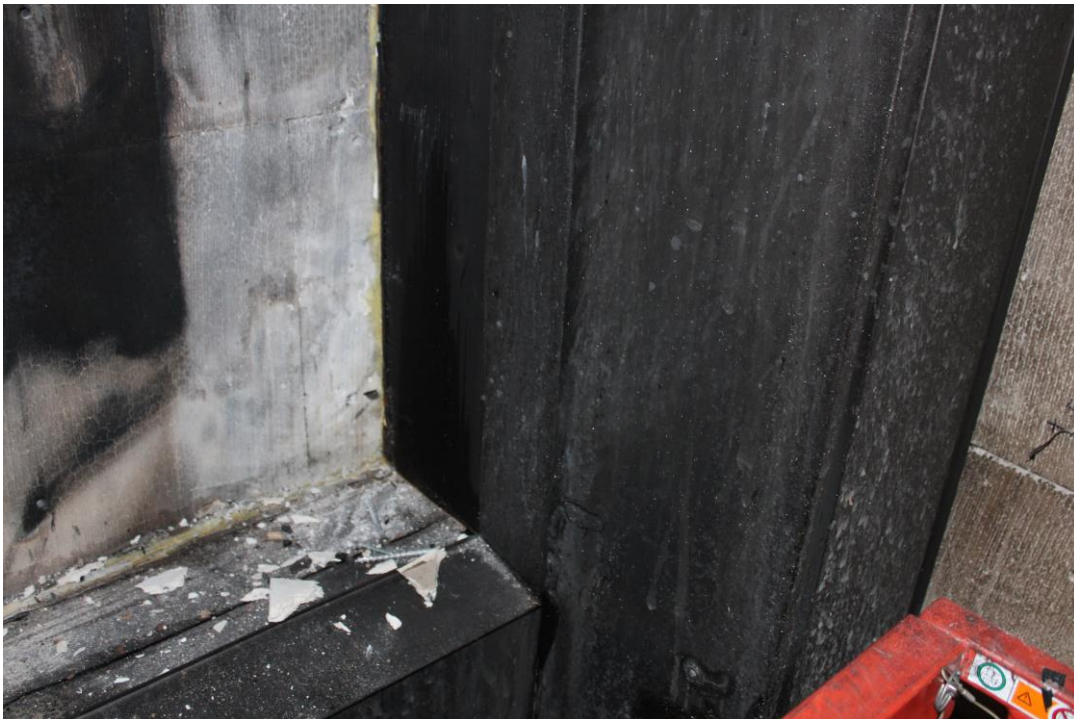
Photo No. 30 Test specimen after the test. Detailed photo of 2. Floor right bottom corner.
