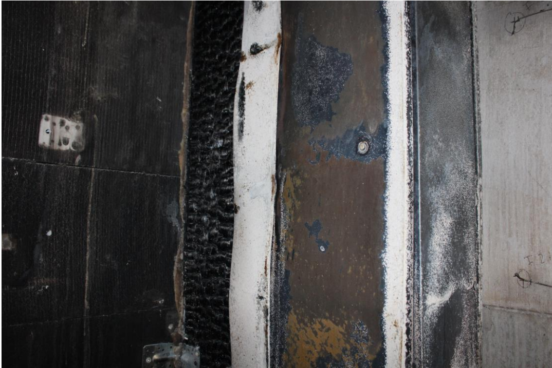
Photo No. 25 Test specimen after the test. Detailed photo of 1. Floor right frame.
