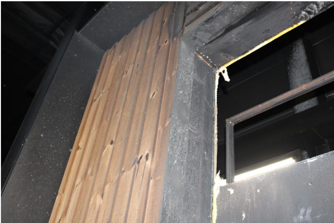
Photo No. 28 Test specimen after the test. Detailed photo of 2. Floor left top corner.
